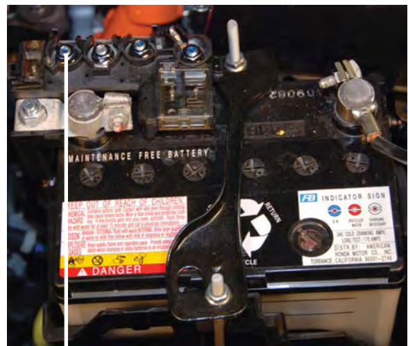
DC to DC Converter Cable Connection
