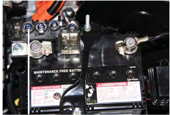
DC to DC Converter Cable Connection
